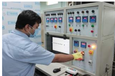
Electrical Safety Test Machine
